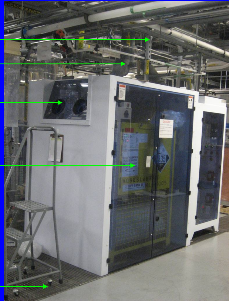
Chemical supply cabinet for 25% TMAH
